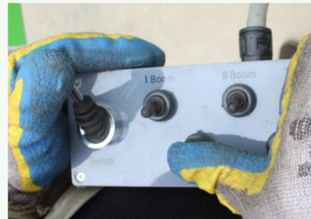
Diesel/Gas Motor are equipped with manual accelerator.
