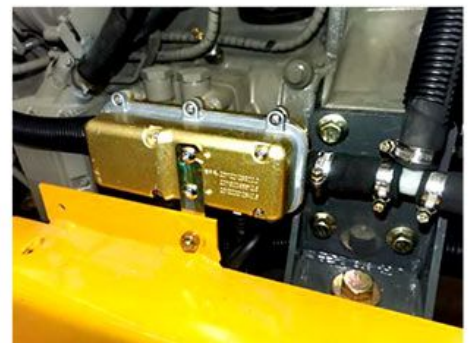
220V WATER PRE-HEATER
